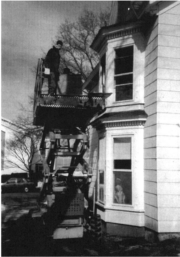
ABOVE: Photo of work being done at the Knight-Sutton Museum, 123 Main St., Akron
